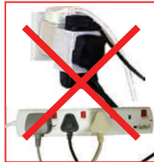
NO MULTIPLE SOCKET/ OWN EXTENSION
